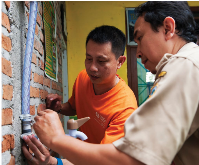
A volunteer and a public health official work together to install a water filter in Lamongan, Indonesia
